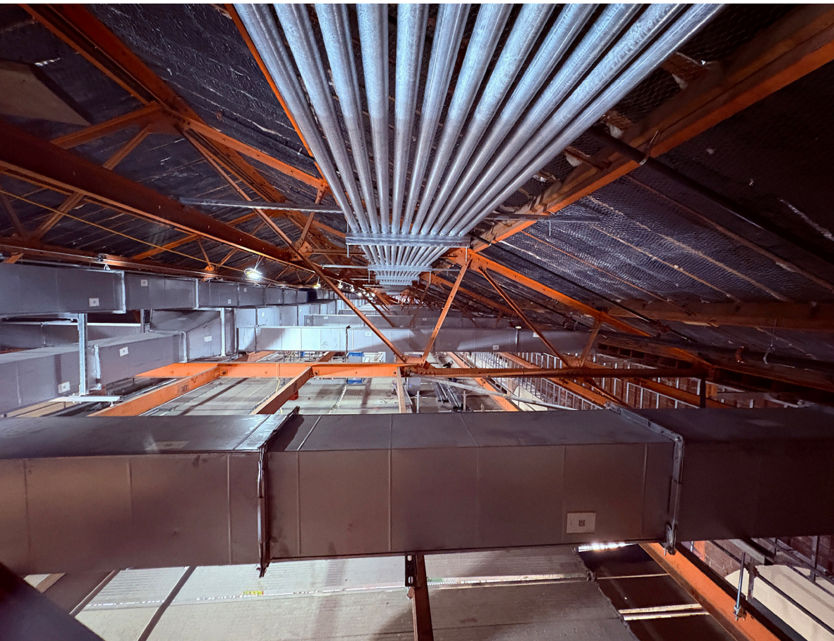
All of the HVAC and electrical work in the rafters have been completed.
